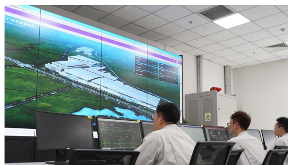
Energy Management System
