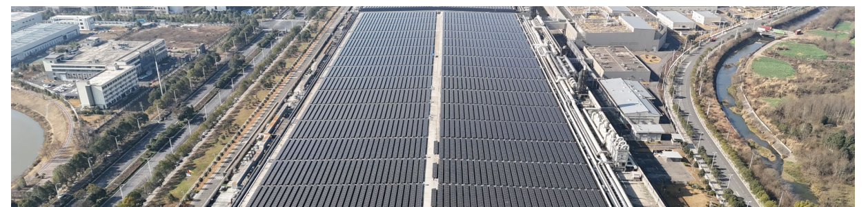
Rooftop Photovoltaic Systems
